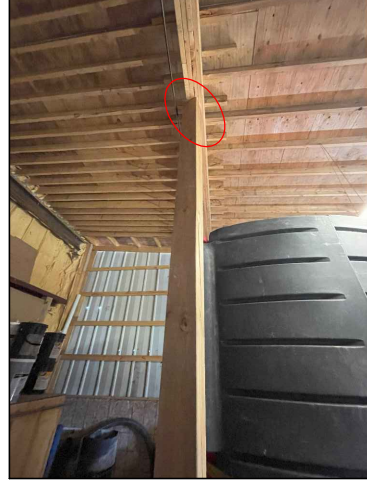
PHOTO 3 WARPED WOOD COLUMN AT BEAM CONNECTION
