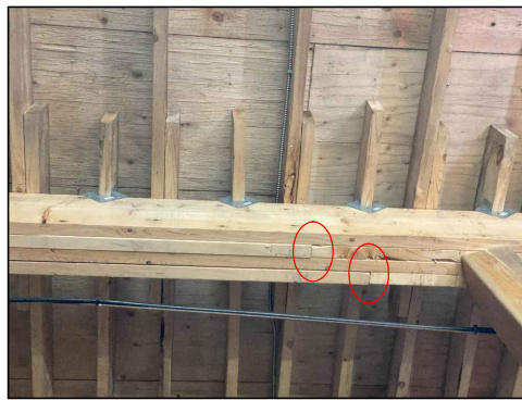
PHOTO 7 BUILT-UP BEAM, JOINTS NOT SUPPORTED BY COLUMN
