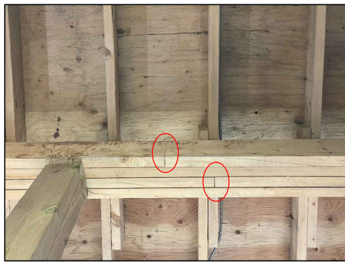
PHOTO 6 BUILT-UP BEAM - JOINTS NOT SUPPORTED BY COLUMN
